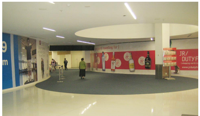
Above: Behind these two hoardings construction teams are beavering away fitting out the two new duty free stores
